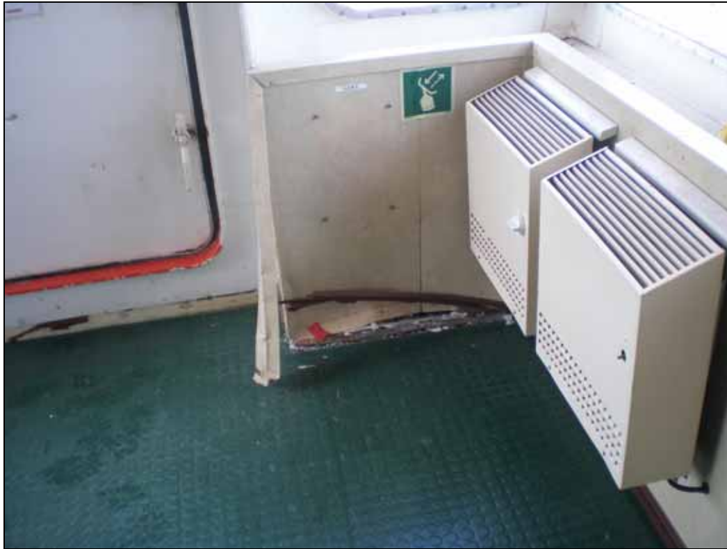
Figure 10: Damage on the port side
