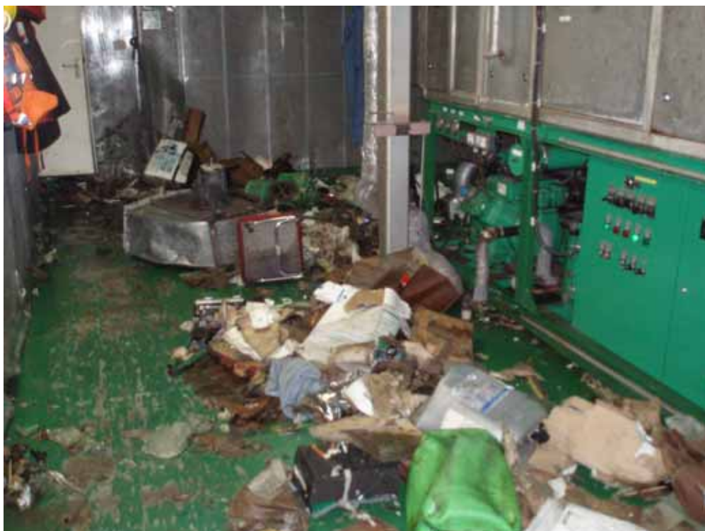
Figure 4: Air conditioning systems compartment
